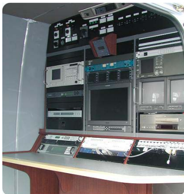
Control desk in side of the VAN. Top part is control of power generator. A Spectrum analyzer is located at left side. Monitors are in the center &
